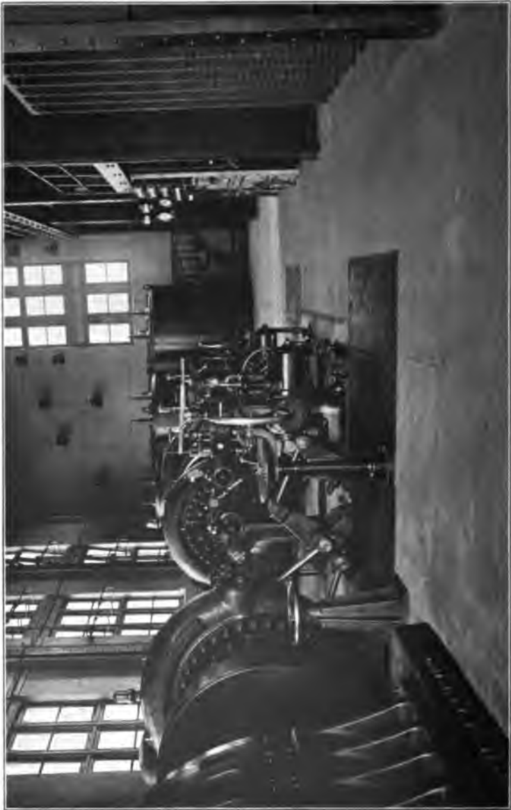
CARP RIVER POWER HOUSE—SHOWING GENERATING EQUIPMENT AND HIGH TENSION TRANSFORMERS.
